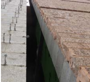
Building / Isolation / Seismic Joint
